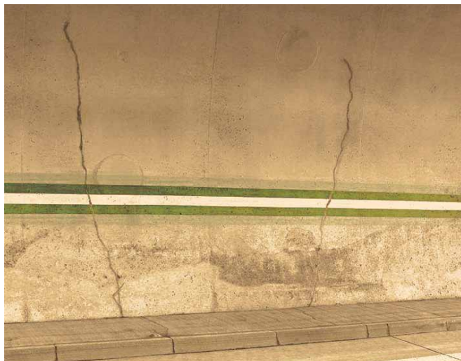
Obr. 2 Trhliny v ostení tunela Horelica Fig. 2 Cracks in the lining in Horelica tunnel
