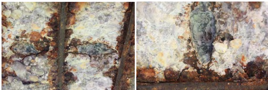
Figure 4 Exposed grouted corroding duct - prestressing reinforcement was free of corrosion at the time of the survey
