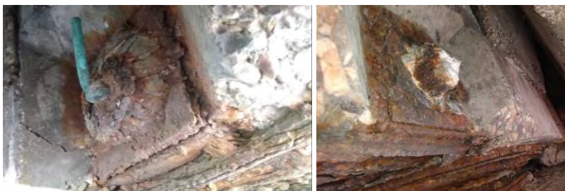
Figure 10 Corrosion on prestressing reinforcement anchors
